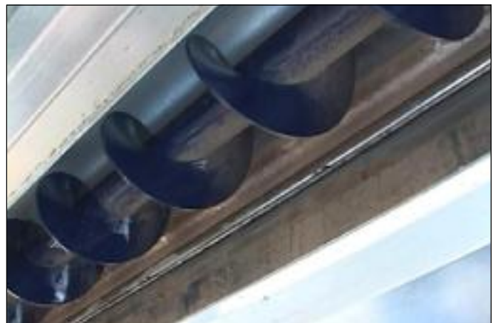
Figure 3.28 - Looking past open cleanout doors at the discharge auger.
