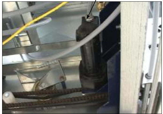
Figure 3.25 - DC Drive Motor with Meter Roll Drive Chain
