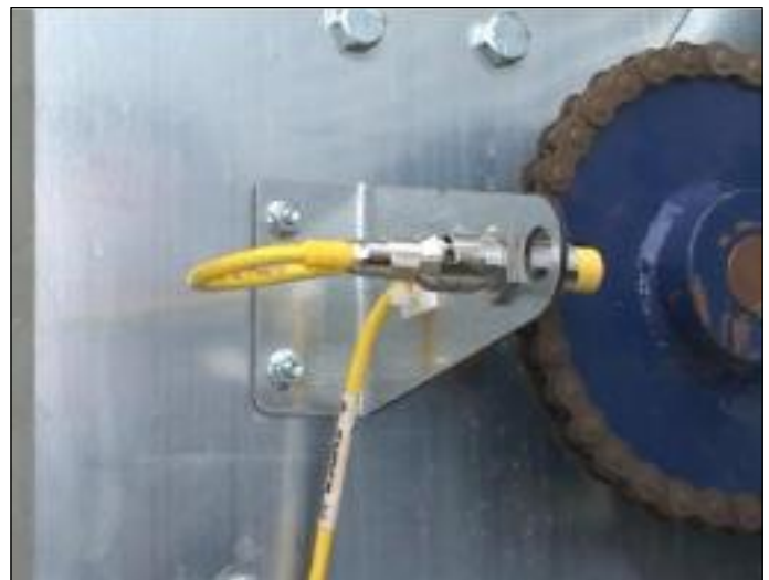
Figure 3.26 - Stall Timer Proximity Switch
