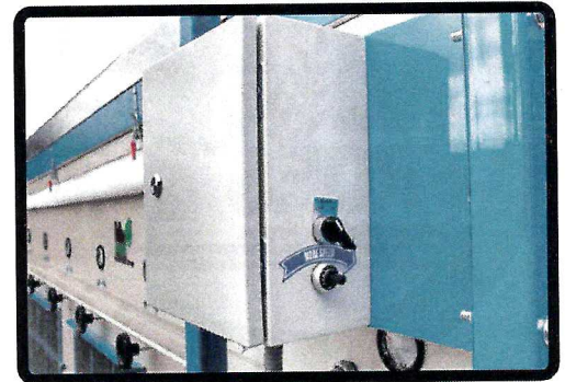
Variable frequency drive Panel
